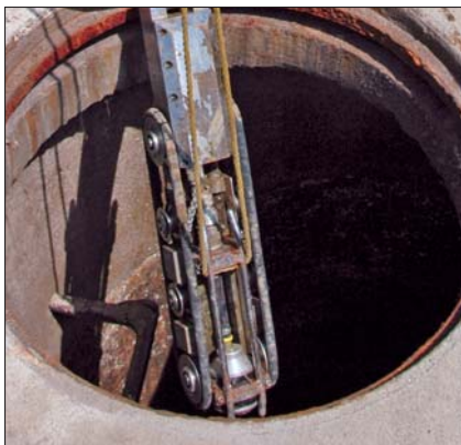
Mr. Rooter of Dubuque deployed its Cyclops crawler camera to inspect a line at the local dog track and casino.
